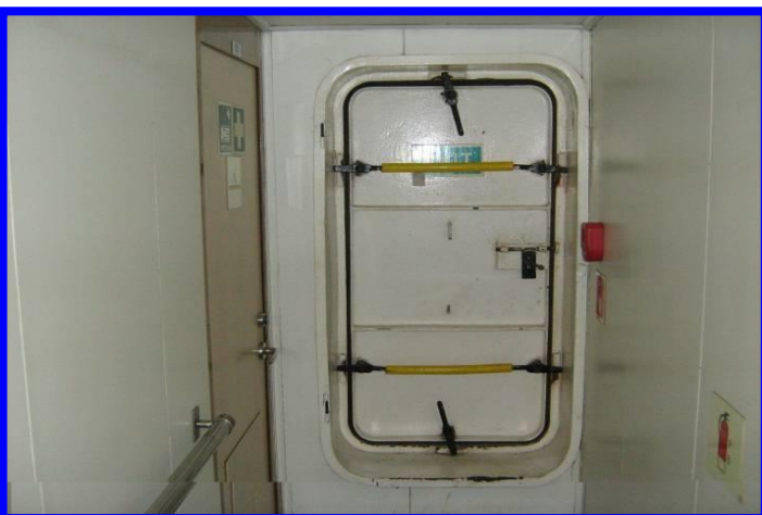
Watertight door effectively secured
