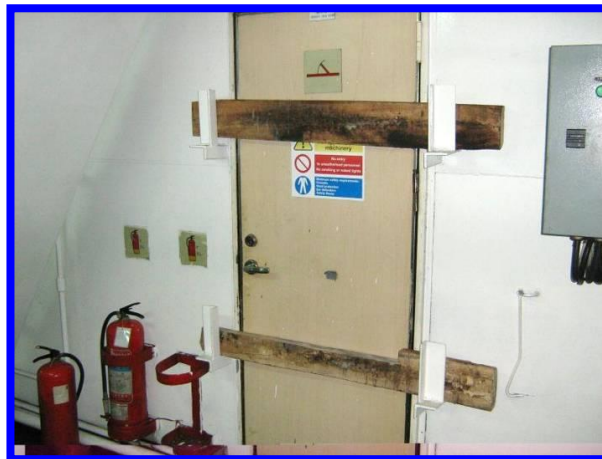
A further deterrent to access should the lock be breached (metal is preferred to wood)
