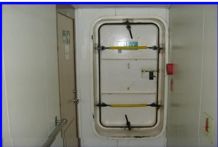
Watertight door effectively secured
